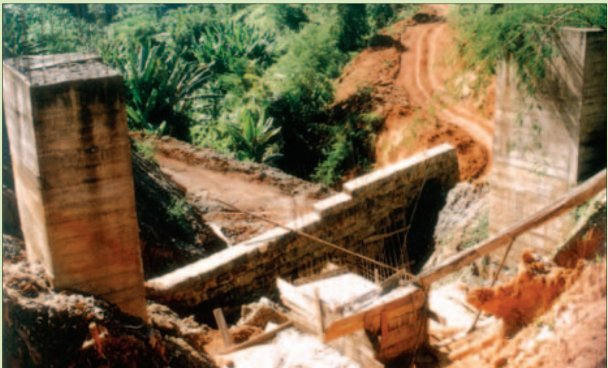
Construction of the Mali Hydro-electric power plant is far from complete; November 2004
