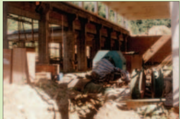
Inner view of the Mali Hydro-electric power plant; November 2004
